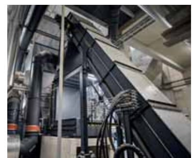
Fuel and primary air supply
