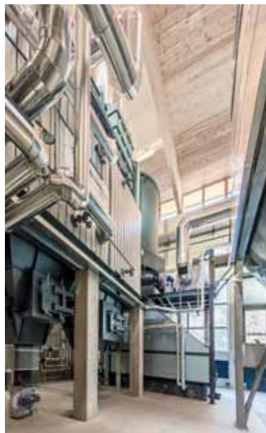
View of the thermal oil boiler and step grate
